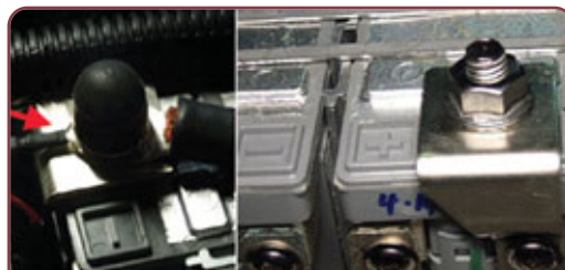
Voltage sensor and cable are attached to the positive terminal (left) and the bus bar is located on the negative terminal (right)
